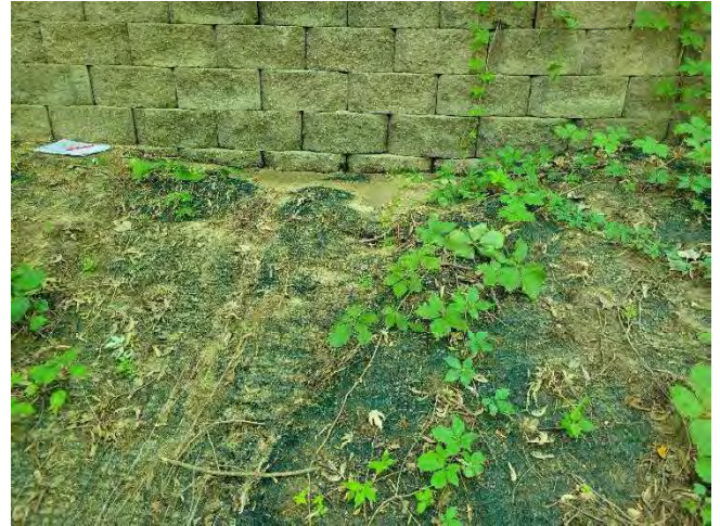
Photo #6: Leakage from retaining wall on east side of ditch, STA: 27+00
