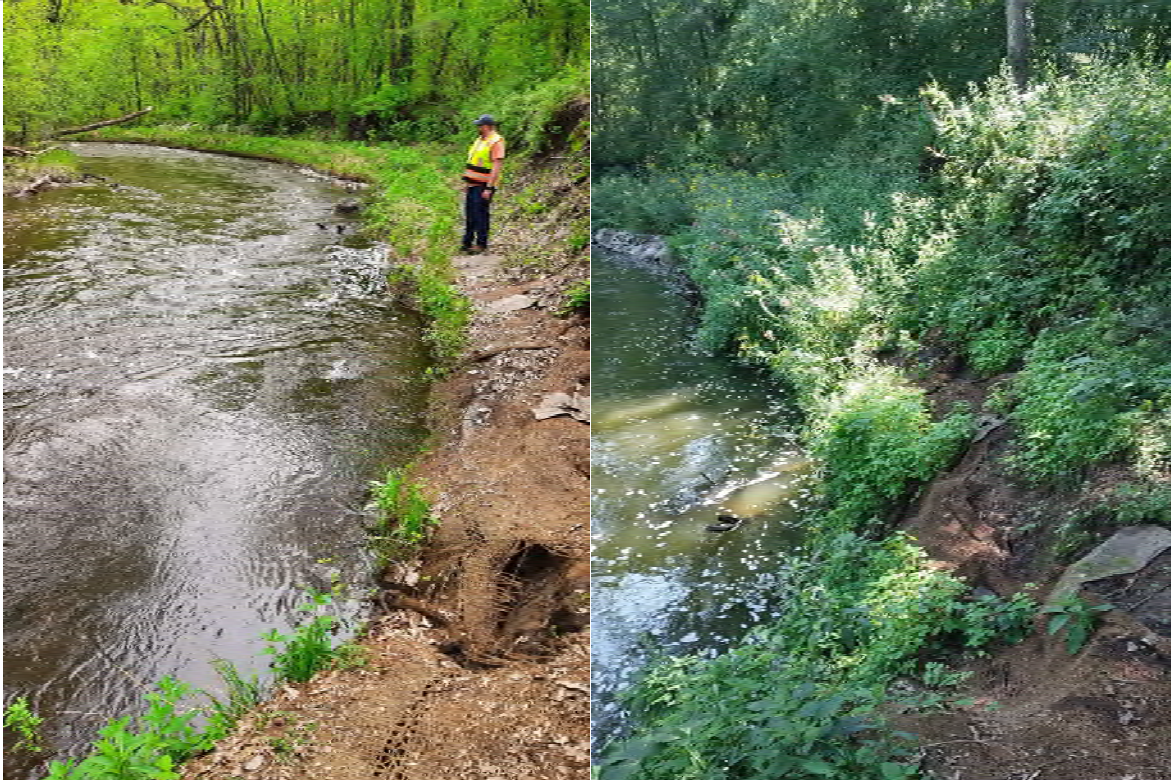
Figure 2. Site 12a, requiring repair. Left: May 2023. Right: August 2023
