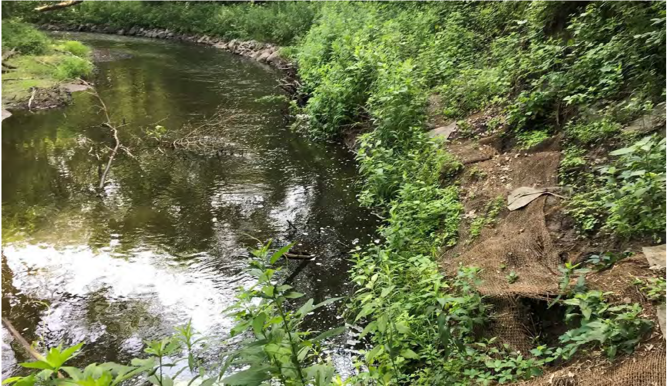
Figure 2. Bank failure along Stabilization Area 12A of the Lower Rice Creek Stabilization project.
