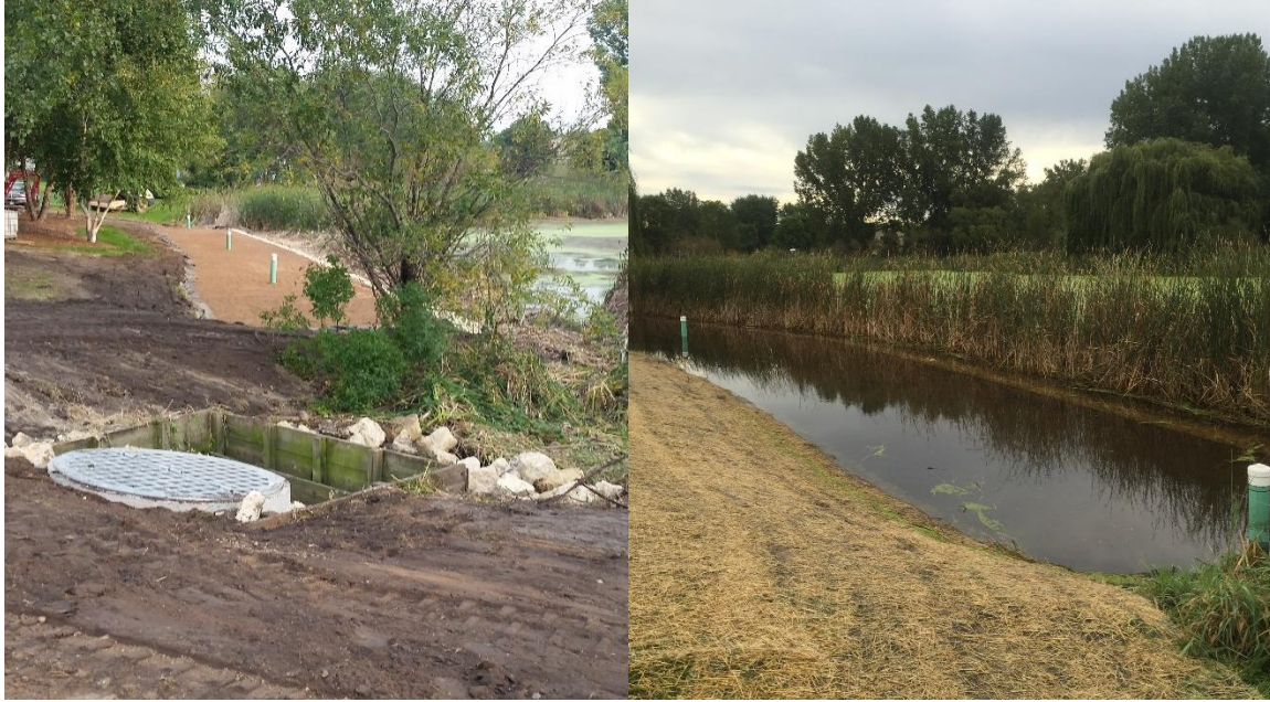
Figure 1. Photos of the Centennial Green IESF. Left: Outlet structure and filter bed during construction Right: Filter bed inundated; water would be flowing through filter and into outlet structure.
