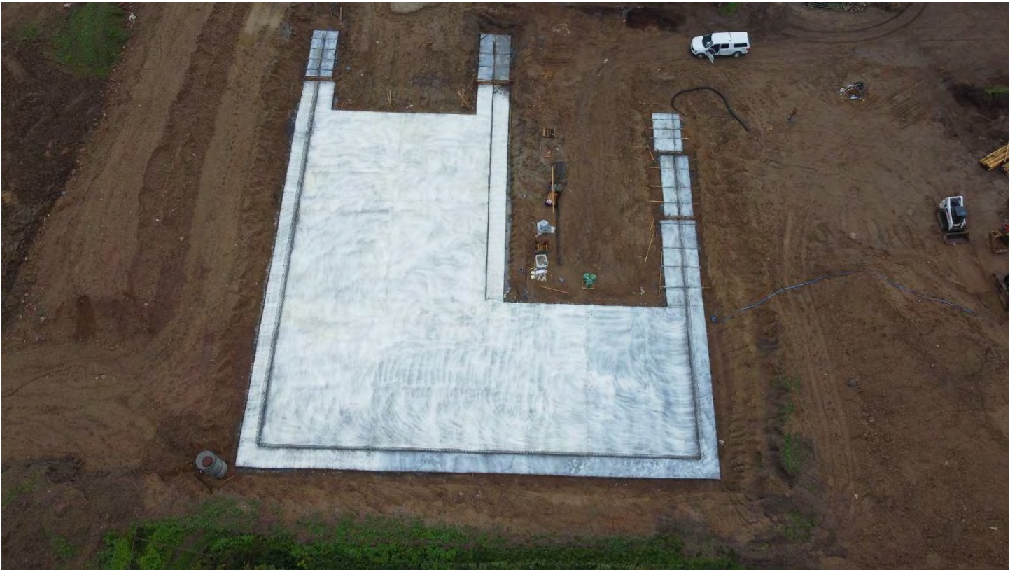
Figure 11 Floor concrete pour 24 hours post pour, crack and visual inspection, pick up QA break cylinders Krcmarik 6/11/24
