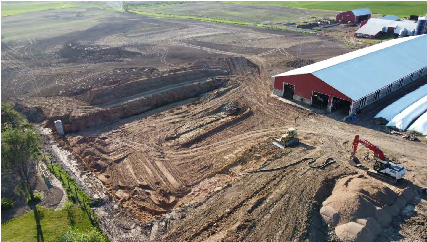
Figure 2 Tile and observation well placed, sand base under construction in final excavation
