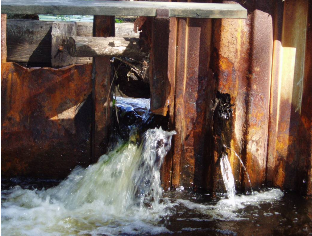
Figure 11. Outlet Weir Corrosion at Farrel's (E-2) Wetland.
