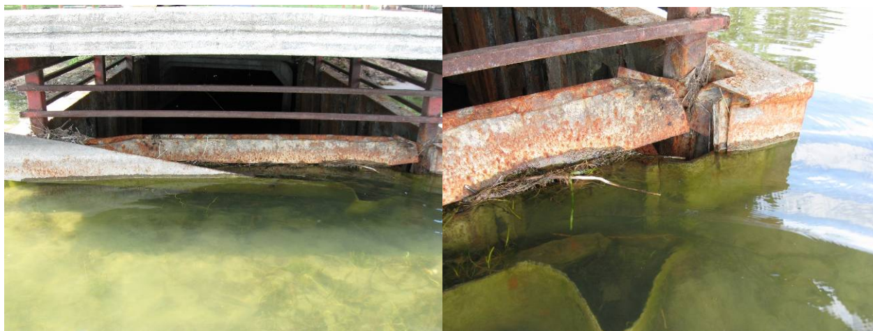
Figure 7. Photos of damaged outlet structure, Sept 9, 2008
